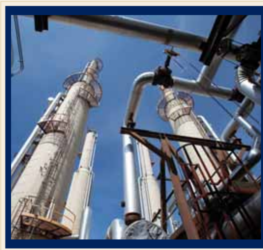
NGL Extraction Facilities, Cochrane, AB.
